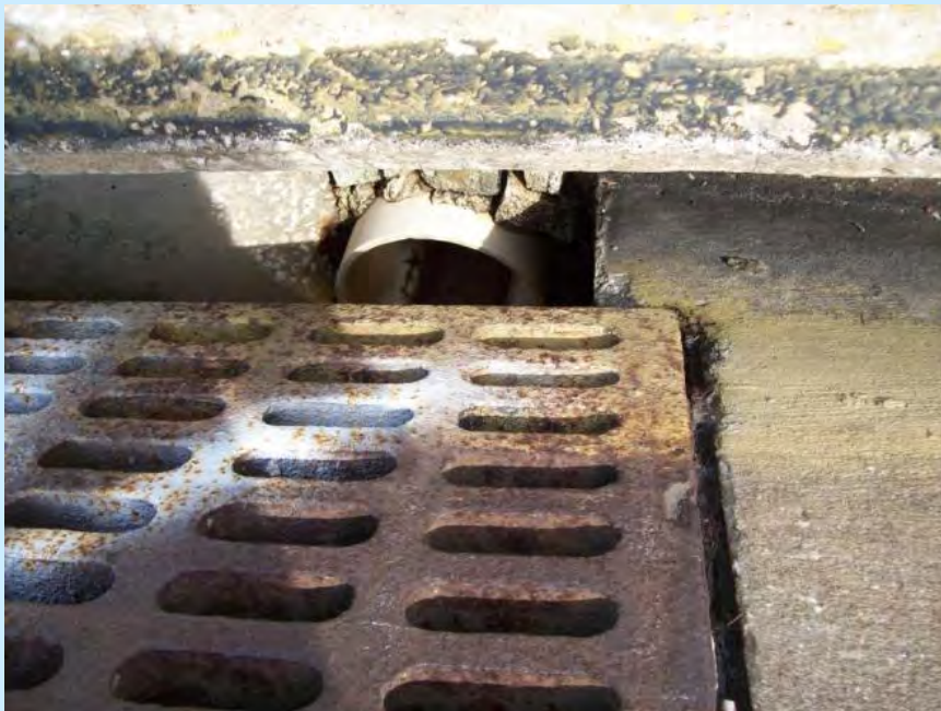
Unknown pipe into storm sewer inlet
