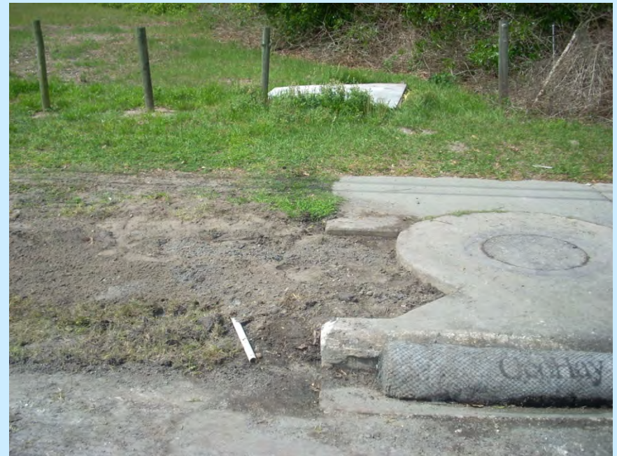
Unknown pipe to inlet
